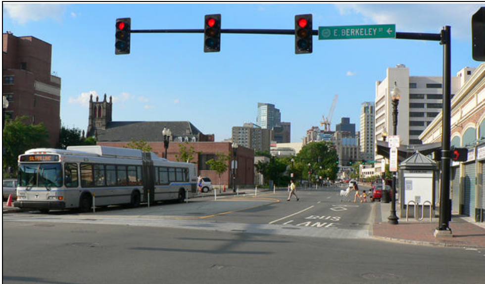
Figure 5: Washington Street at East Berkeley Street After Construction (Outbound bus is operating in contraflow lane obtained by removing parking and moving the curb. Note inbound bus stop on right)
